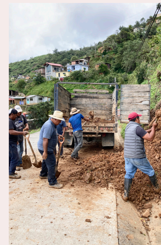
Men doing communal labor ( tequio ) to clear a landslide
